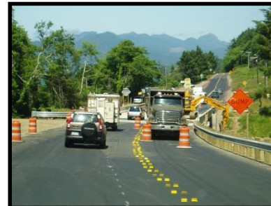
MO – Maintenance & Ops
